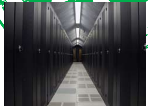
Through both hot- and cold-aisle containment practices, we maximize cooling efficiency in our data centers.
