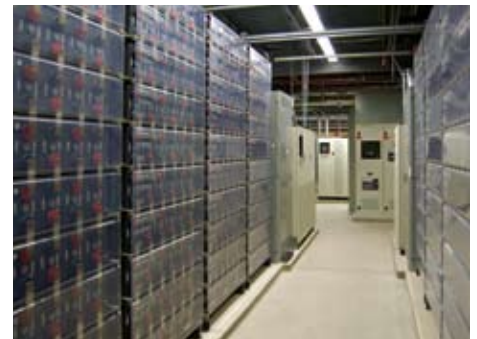
Utilizing our long-lasting recycled battery string greatly reduces our environmental impact.
